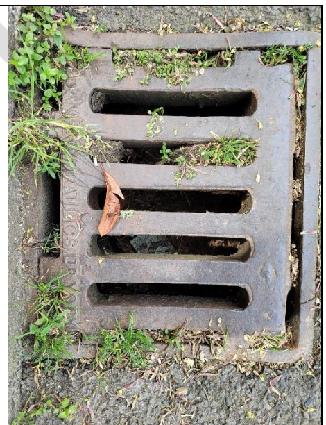
Figure 10: Gully on Blind Lane
