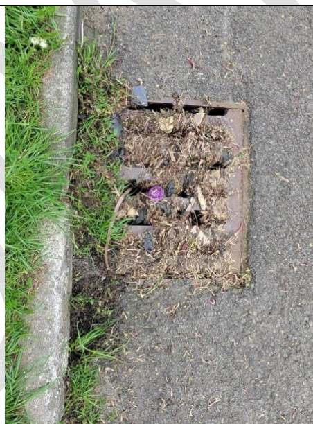
Figure 9: "Blinded" Gully on Blind Lane
